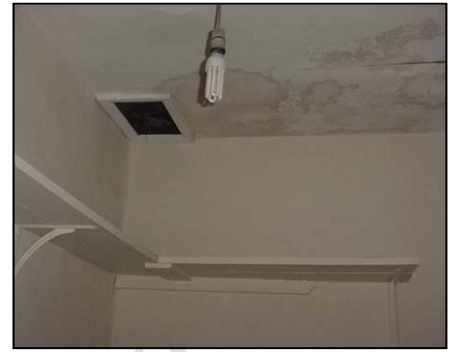
Dampness above staircase area
