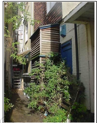
Rear view- shiplap boarding needs re-staining
