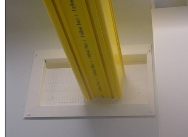
High Level trunking barrier
