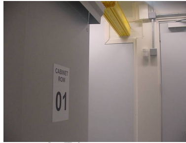
Conduit at high level
