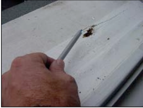
Wet rot in the sliding sash window
