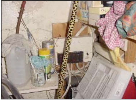
Dated fuse board
