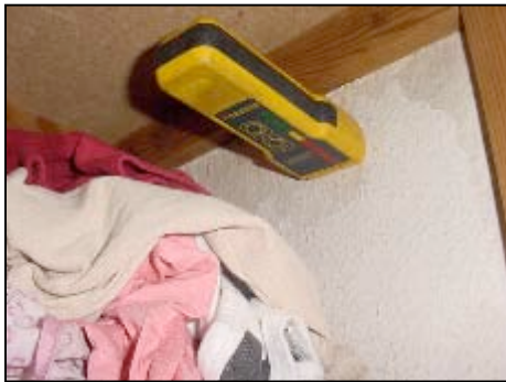
Dampness coming in through the walls
