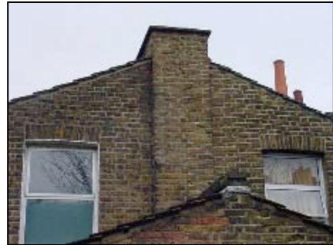
This is the rear view of the chimney where you can see some re-pointing has taken place.
