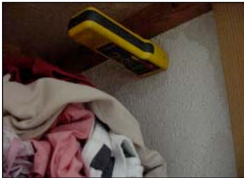
The dampness found within the cupboard
