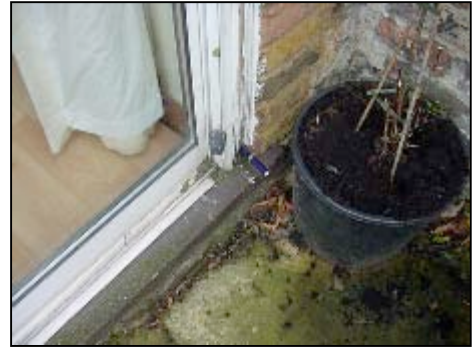
This is the base of the rear doors
