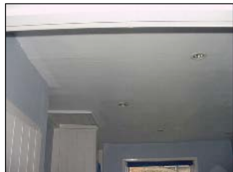
Ceiling Lights set within the bathroom
