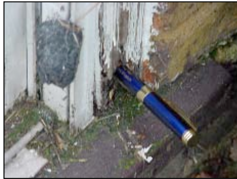
This is a close up of my pen pushed into the rotten timber
