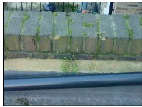
A close up of the parapet wall reveals that there may be some dampness getting in but this is likely to be minor (the correct detail for this is to have a capping stone on top of the brickwork to stop rain getting in from the top).
