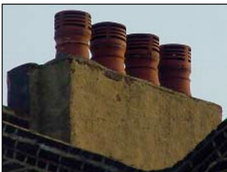
A photo of the chimney taken with a x16 zoom camera lens.
