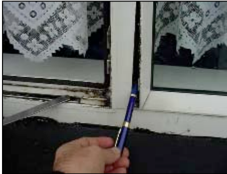
Some of the window beads are loose.
