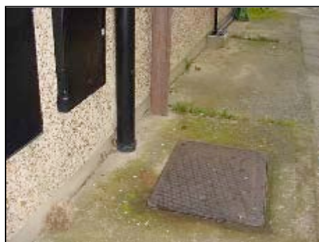
Inspection chamber close to the house
